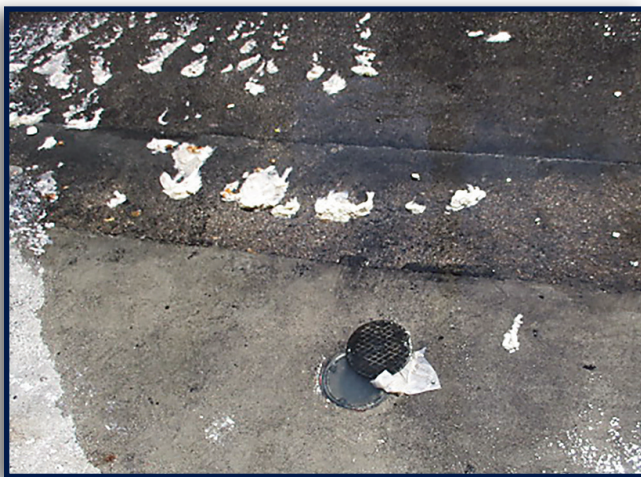
Fig. 2: Raw sewage, pieces of toilet paper, and other solids spilled out of a clean-out. The raw sewage and solids brought to the surface contaminate roads, streets, and Lake Mead.
